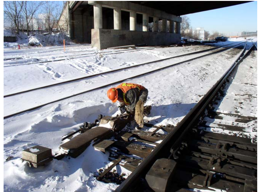
Main Line Interlocker
